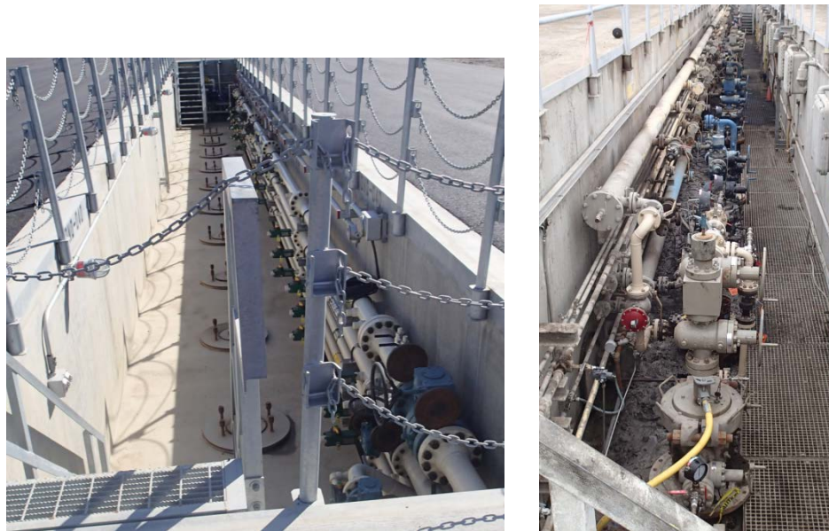
Figure 2: Typical Common Well Cellars
